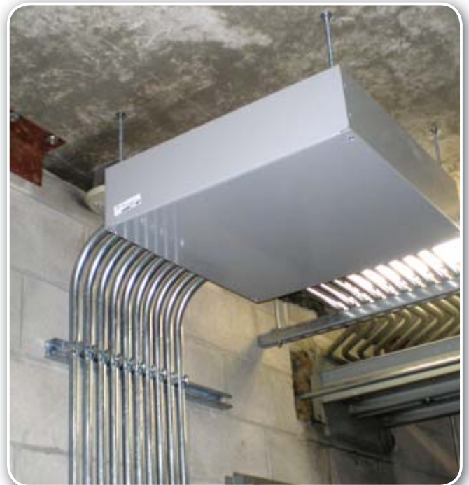
A San Diego condominium tower installed wiring hubs on each floor of the parking garage to accommodate charging station installations at residents' individual parking places. See the case study in Plug-in Electric Vehicle Charging Infrastructure Guidelines for Multi-unit Dwellings . See Additional Resources.
